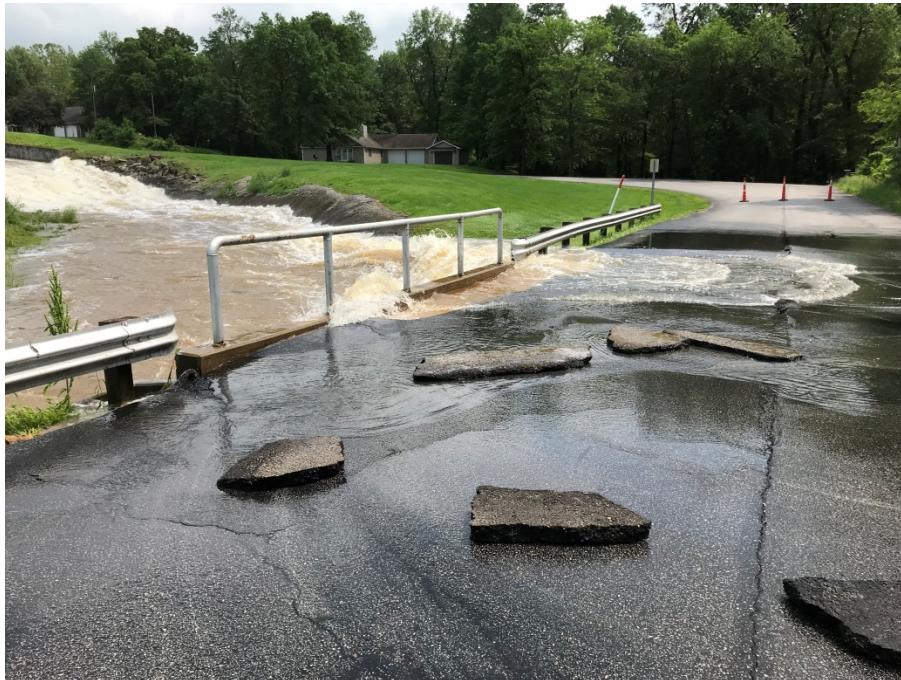
Damage in Lamar as a result of flooding from the May 2019 storms
